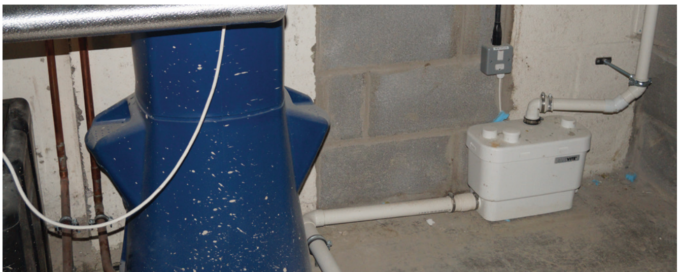
A Sanivite discharges water that is tested weekly to ensure there is no contamination in the side stream filters
