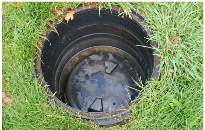
The Saniflos is installed in a 1m deep hole and topped by a manhole cover that is flush with the grass.
