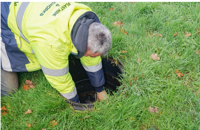
Access to the Saniflos is very simple. Once the manhole cover is removed it just takes a few screws to loosen the Saniflos lid to gain access to the motors.
