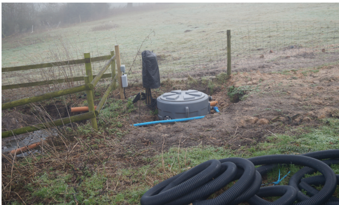
The Saniflos 610 in-situ. Landscaping will cover all but the lid in due course
